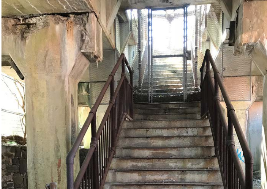
Fig. 44: The Derelict North Shore Railroad Viaduct and Rail Line
